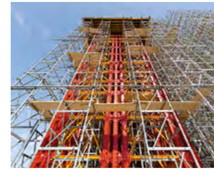
Bundled 42-leg VARIOKIT shoring towers carried the extremely high loads in the connecting area of the steel arch connections.
