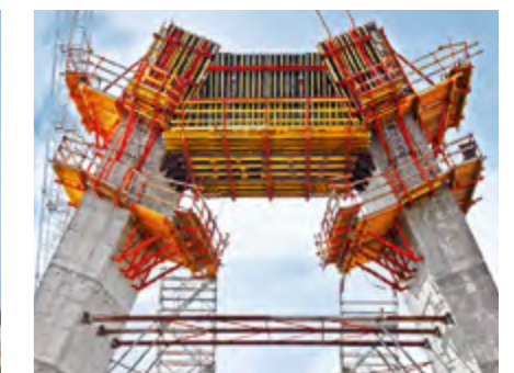
The formwork for the vertex arch was formed with the VARIO GT 24 girder wall formwork system and stored on internally mounted special brackets.
