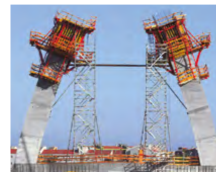
The SKS climbing scaffold could be optimally adapted to suit the complicated pylon geometry. Accessing the work platforms was carried out through PERI UP scaffold stairs.
