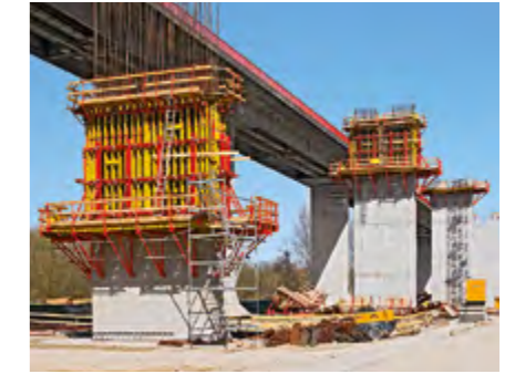
With CB/VARIO climbing formwork units, the 40 piers of the foreland bridge could be cost-effectively constructed.
