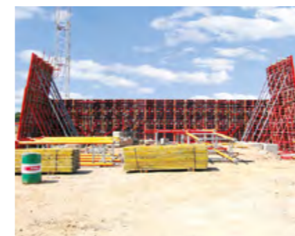
The bridge abutments were formed with TRIO, the curved wall surfaces with RUNDFLEX. With the BFD alignment coupler as the only connecting part, the two systems could also be combined with each other.
