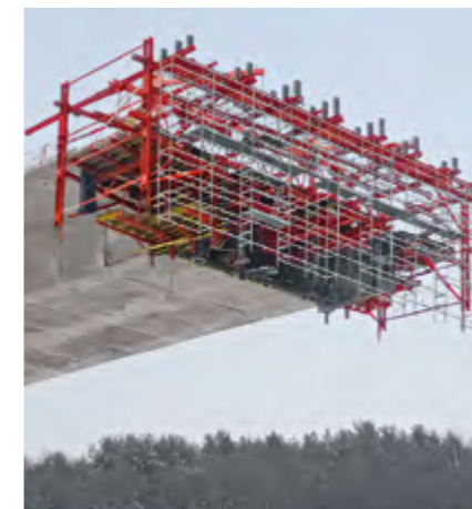
For safe working platforms and access, VARIOKIT and PERI UP could be ideally combined.
