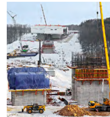
Apart from the VARIOKIT balanced cantilever equipment, the CB/VARIO climbing formwork was also an important part of the PERI project solution.
