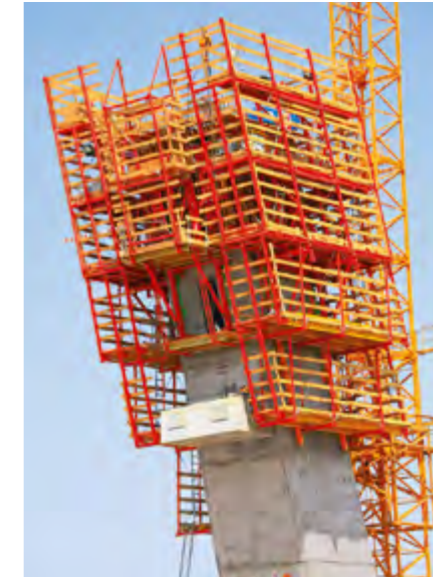
The five working levels provided safe and generously-sized working areas for personnel, tools and equipment.
