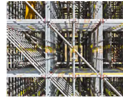
By halving the 150-cm basic grid using 75-cm long ledgers, the PERI UP could be optimally adapted for the load concentrations.
