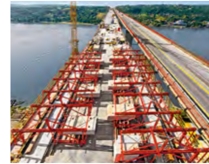
Two groups of VARIOKIT formwork carriages worked simultaneously – for realizing the weekly completion of six casting segments.
