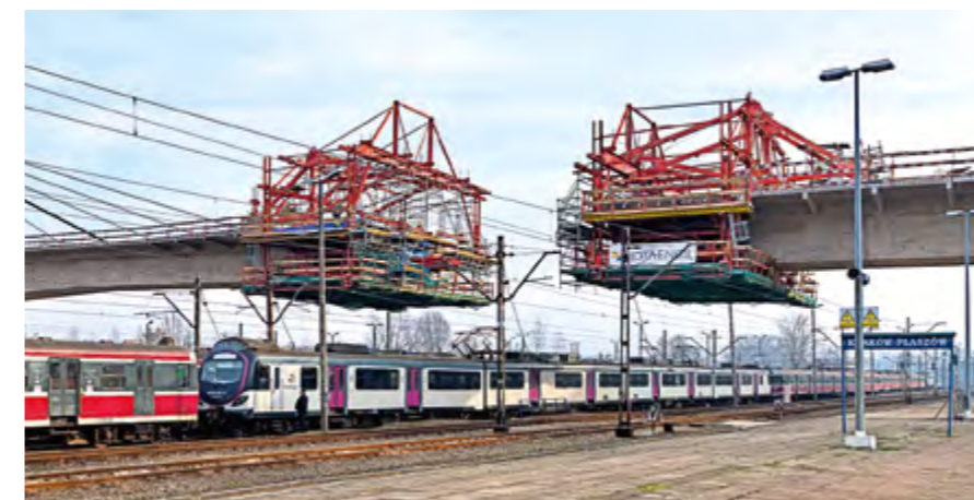
General Contractor Mota-Engil Central Europe S.A. Field Service PERI Poland – Krakow Office, Kattowitz Office
