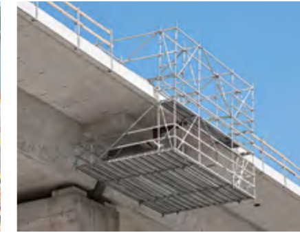
PERI UP suspended scaffold served as safe access means to the bearing points on the pier heads.
